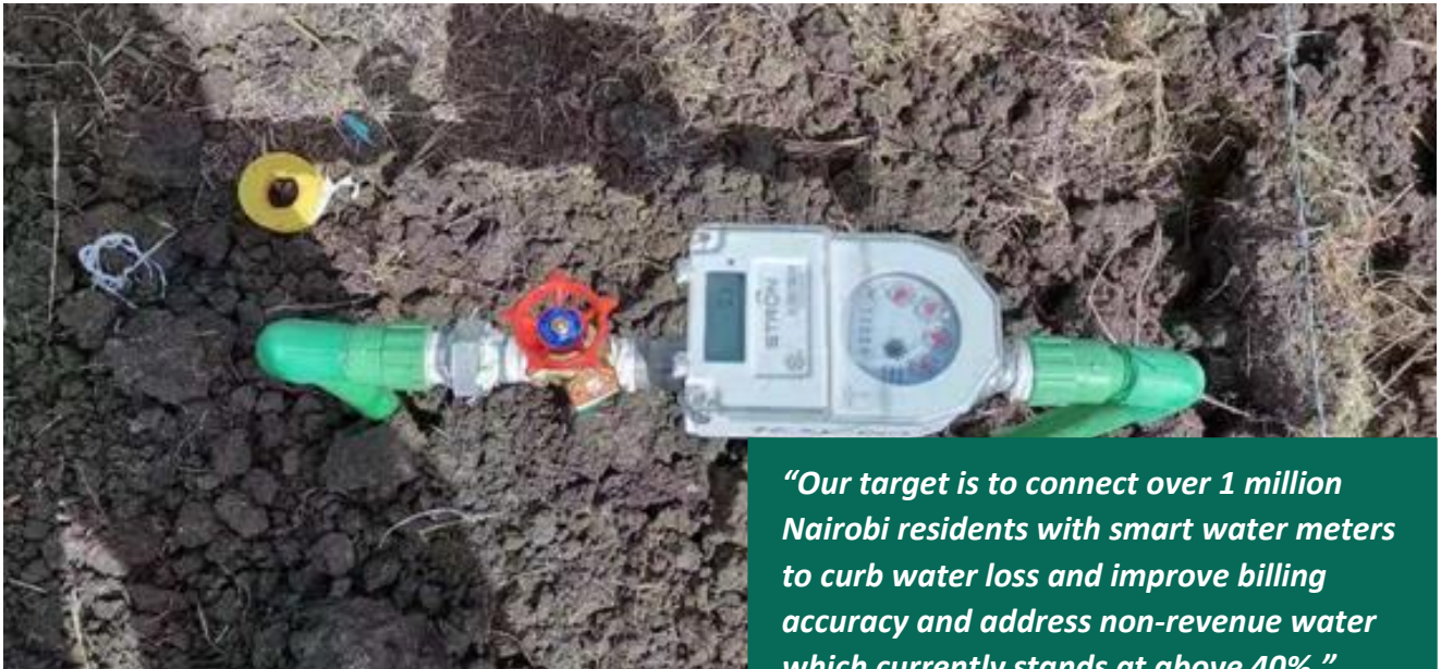
Figure 5: Smart water meter
